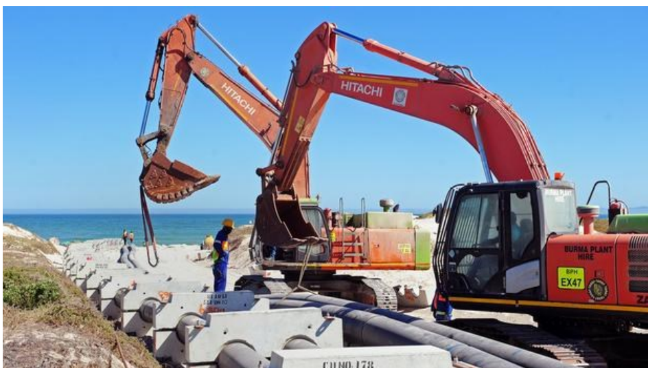
Construction is under way on a desalination plant at Strandfontein Beach. This plant will be one of several to supplement the City of Cape Town's fresh water supply. Photo: African News Agency.
